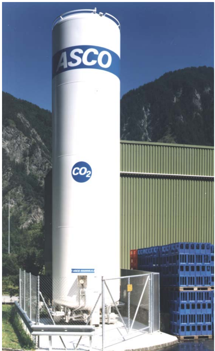
37 t vertical ASCO CO 2 - Storage Tank, vacuum insulated
